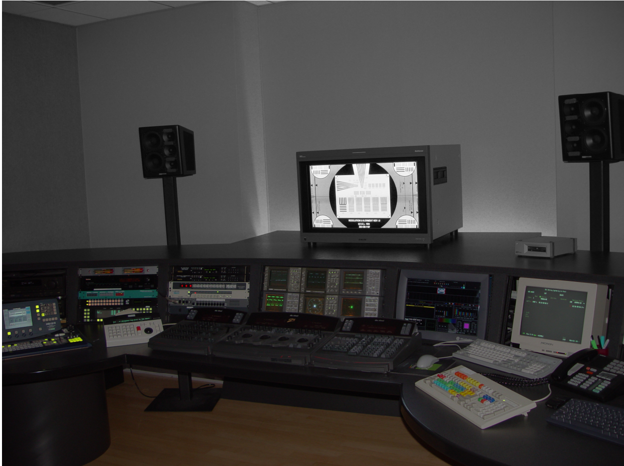
Telecine Bay where the lights have been turned up so you can see the equipment in the room
